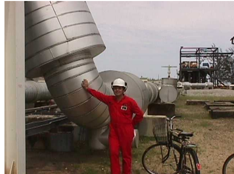
Compressor Plant & Chilled Water Piping (EPS Works-as Project Engineer (Year 1998) Construction)
